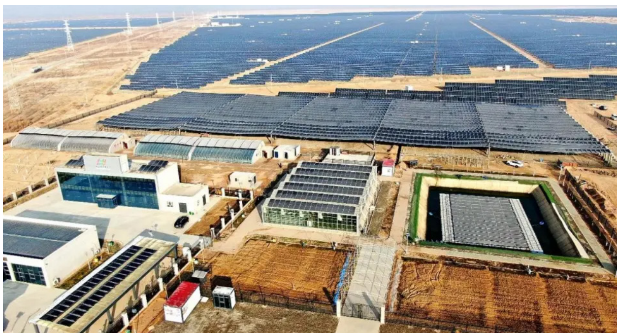
Figure 8: Photovoltaic project close to Aral City, Xinjiang 89
